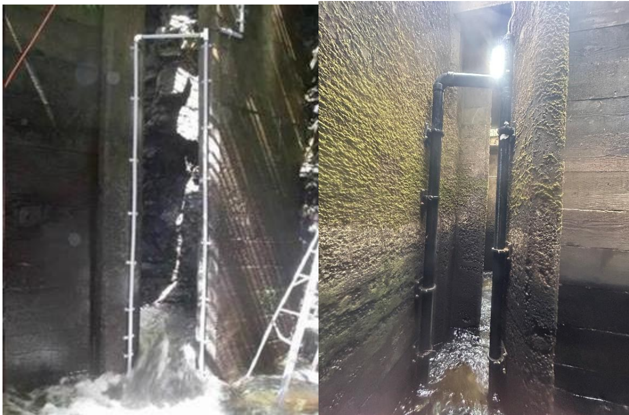
Figure 3. PIT antenna array installed at the Stamp River fishway showing the upstream antenna (left) and downstream antenna (right).
